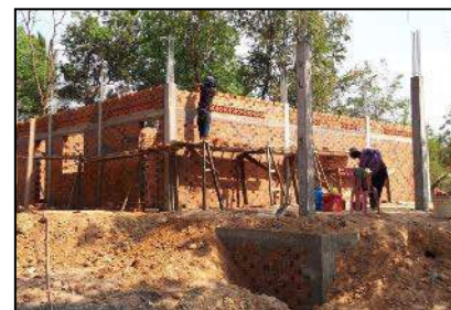
Front view—classrooms out front will be covered, but largely open air spaces.
